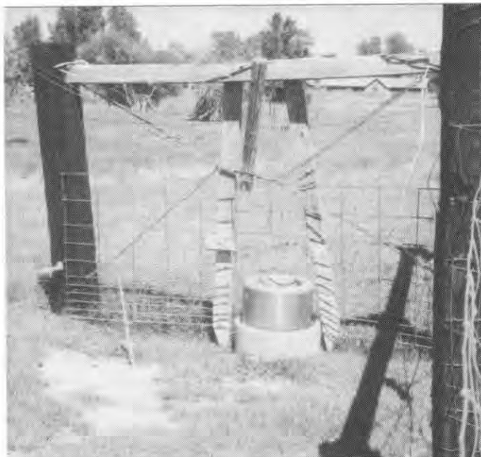
The ultimate watering bucket? Automatic waters, placed under a fence to service two paddocks. It's warmed by a heating element and fed by buried water pipes—low maintenance and freeze proof! Photographed at the Dooling ranch.
